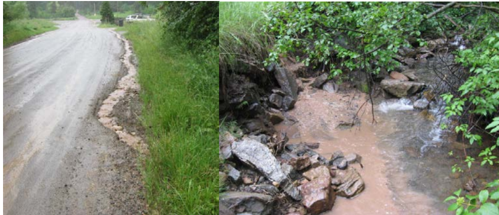
Figure 5-3. Road erosion and associated sediment loading to Bear Creek observed in 2009.
