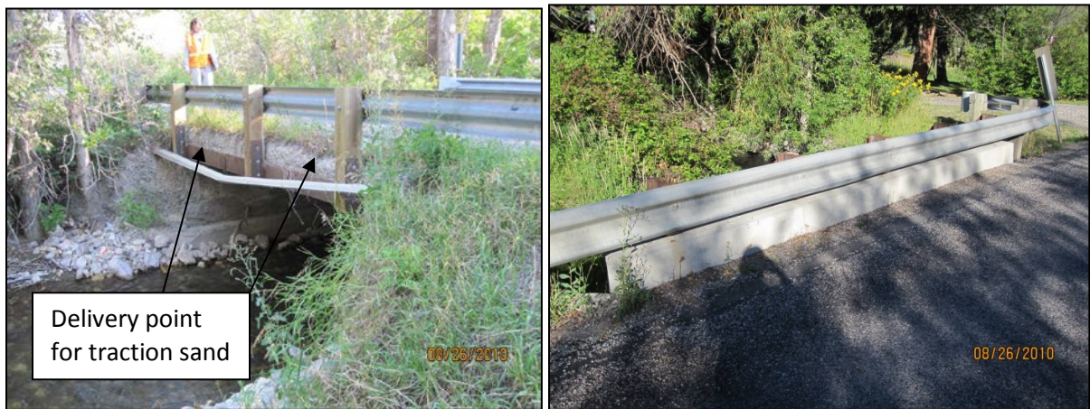
Figure 5-4. Crossing with observed areas of traction sand delivery (left); curbed crossing (right).
